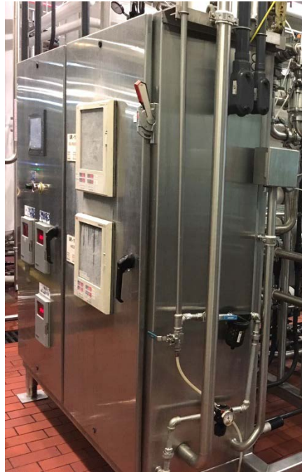
Figure 6 Control Panel Reference Image
